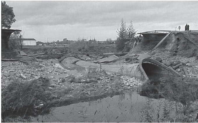
Fig. 2 – Road and aqueduct destroyed by unusual flood.
